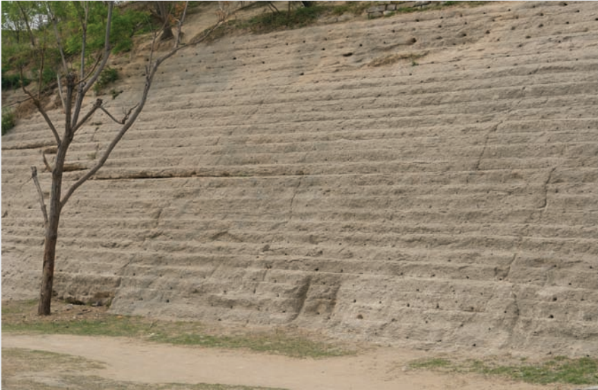
The inner wall at Kaifeng was not clad in brick, and reveals the successive layers of rammed earth along its sloping side.
